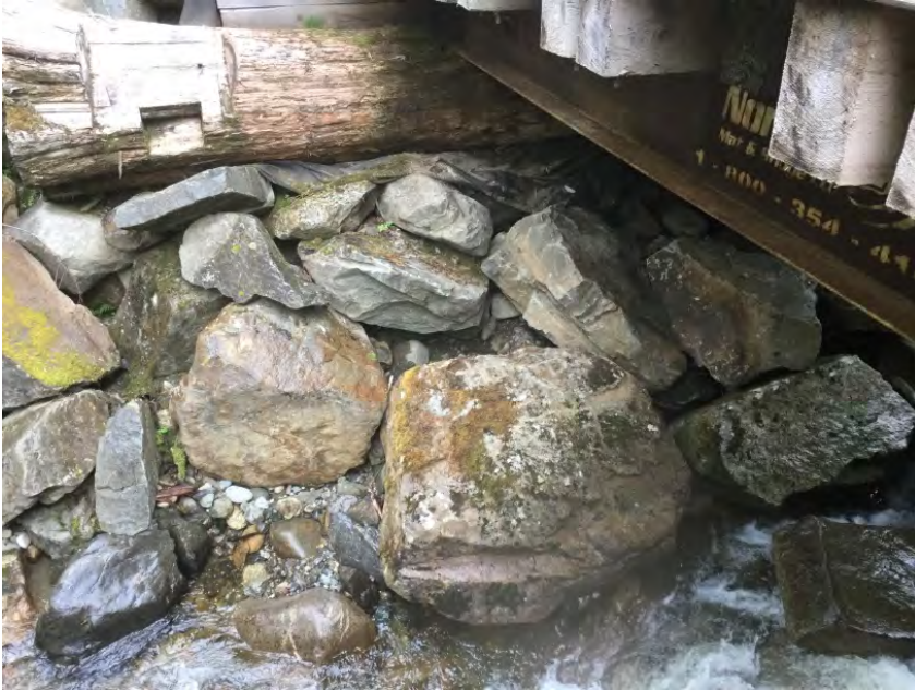
Riprap not well keyed/tied together
